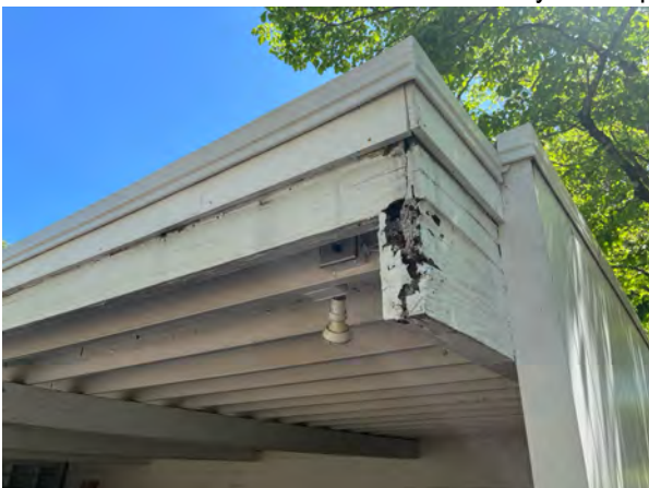
Example of rotted wood in need of repair and replacement. This work is included in the carport repair and restoration project.
