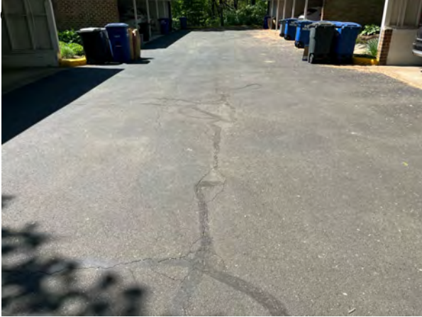
Asphalt pavement is in good condition; however, open cracks need to be sealed to minimize asphalt and base damage. See our recommendations in comments section to maximize pavement useful life.
