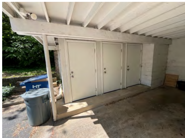
As needed replacement of storage room doors is also included in the reserves.
