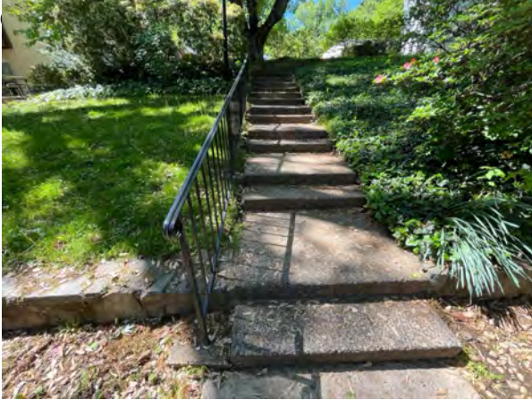
Railings need to be painted to protect against corrosion and post mounted in concrete need to be sealed to prevent standing water from corroding posts.
