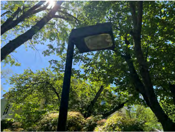
Entry for street lights considers poles, wiring, fixtures and controls will be repaired as needed. No assumption all units will need to be replaced at the same time.
